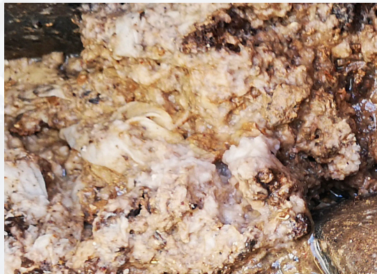
Waste from non-flushable materials causes clogs and ragging problem in pipes and pumps.
